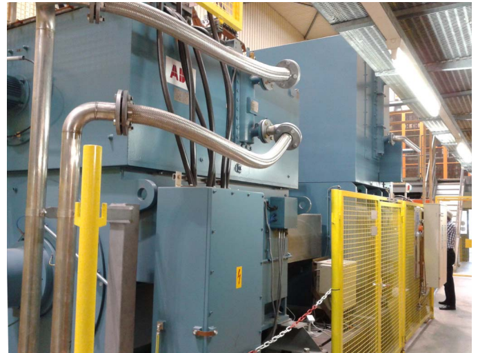
Fig. 5: Test bench for medium voltage drives
