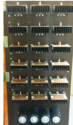
Figure 7. The heatsinks layout of phase U, V and W. Every phase has 6 heatsinks that are arranged vertically
